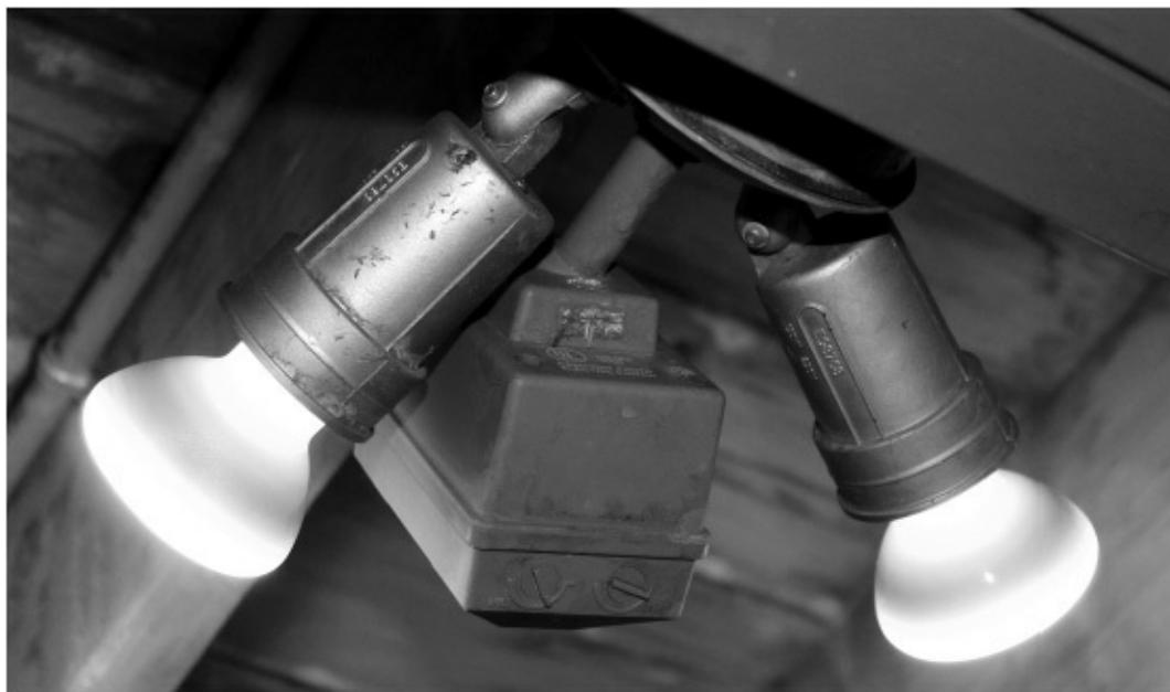
FIGURE 8-1 This photograph shows two 50-watt incandescent spot lights with a motion-sensing actuator between them. It's mounted under a deck, over the back entrance to a residential home.
