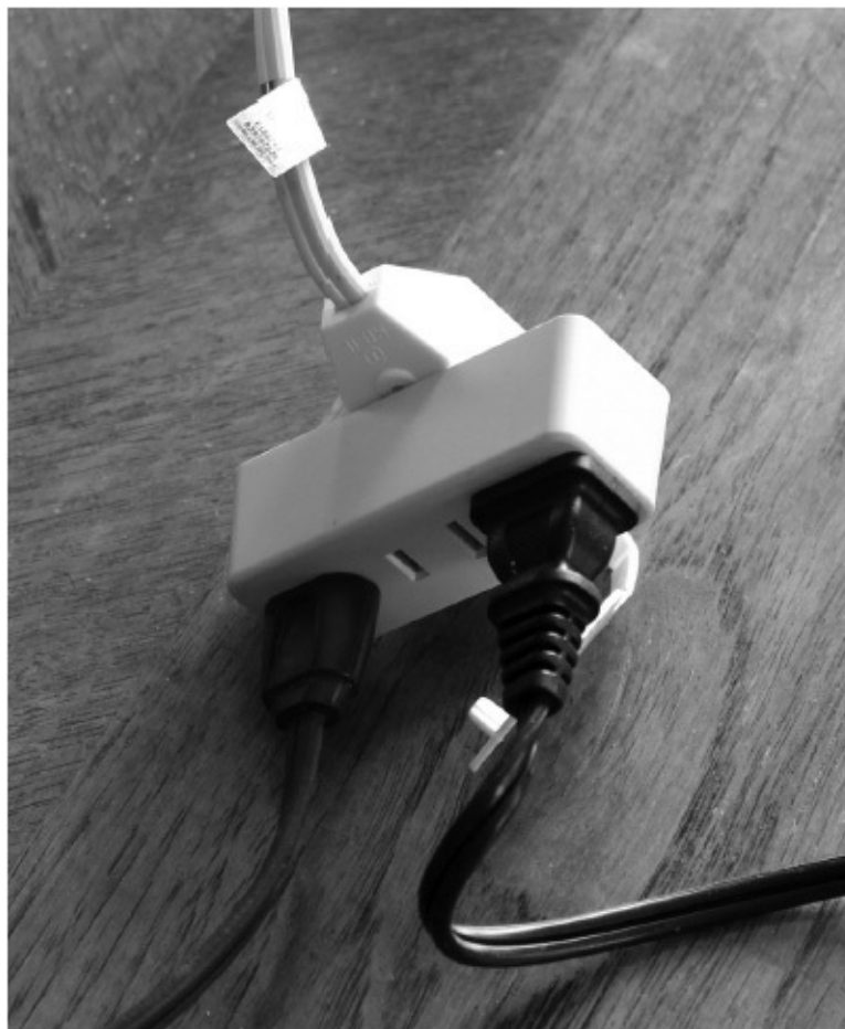
FIGURE 3-10 Improper use of a block tap. Never cascade load-splitting devices one after another like this!
