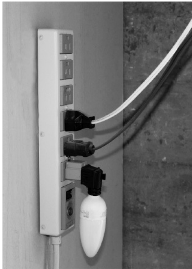
FIGURE 4-3 Power strip for the cords leading from the generator to the computer workstations. The cords lead to uninterruptible power supplies (UPSs).
